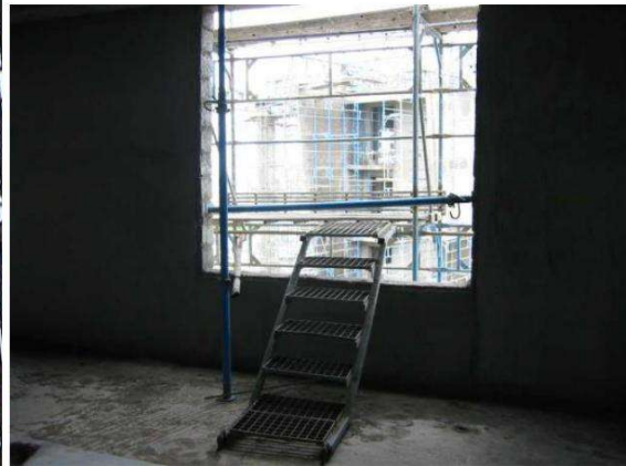
Proper Access to workplatform
